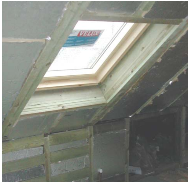
Fig. 1 Fire escape window
