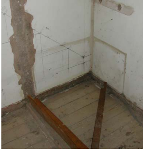
Fig. 2 Staircase opening with the area marked by architect and contractor
